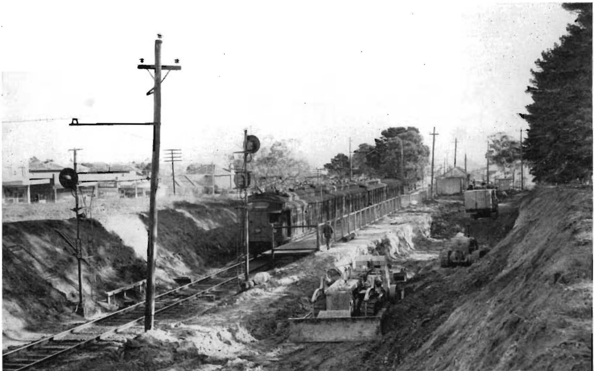
Widening a cutting at Jordanville for the duplication of the Glen Waverley line.
